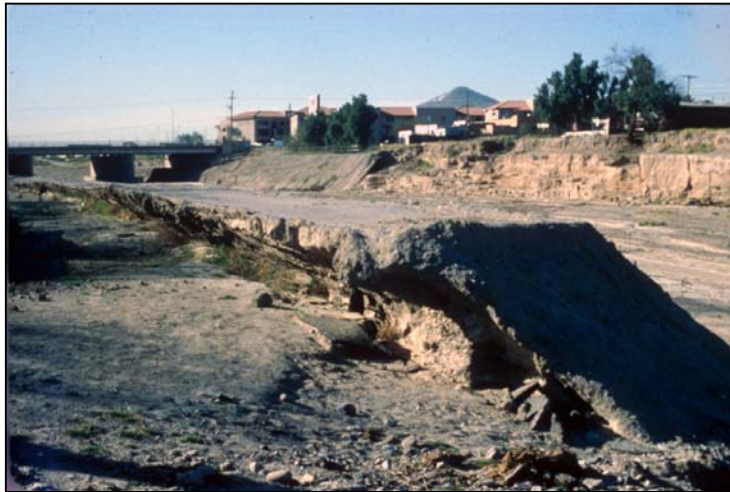
Figure 22. Downstream end of overtopped soil-cement along the Santa Cruz River
