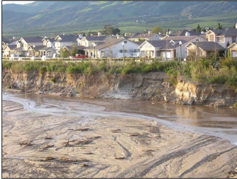
Figure 14. Erosion of bank at Fillmore, CA exposed some buried soil-cement
