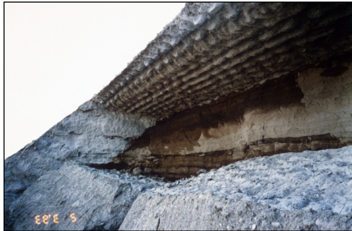
Figure 17. Settlement of Soil-Cement Bank Protection on Santa Cruz River, north of Tucson, Arizona
