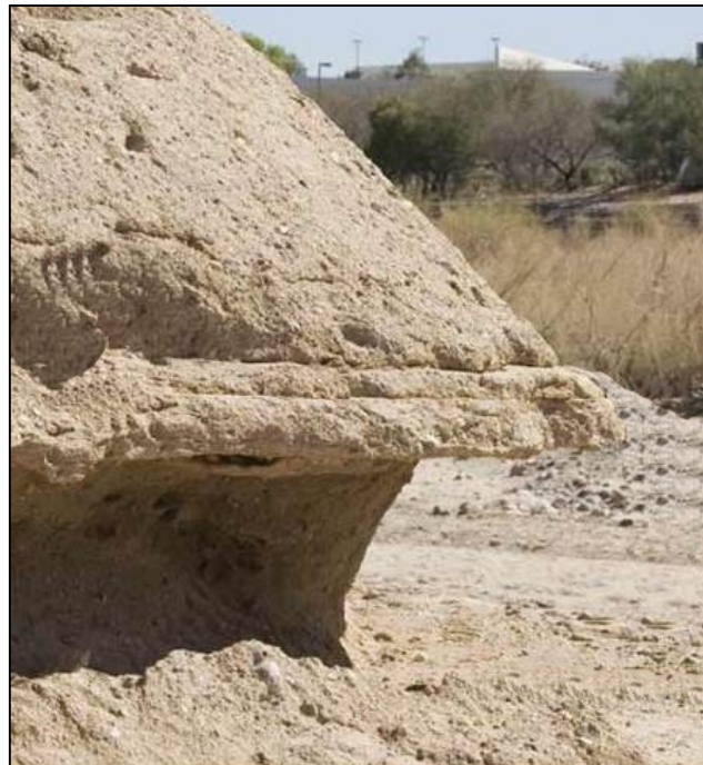
Figure 11. Under cutting of Soil-Cement along Rillito River (2006)
