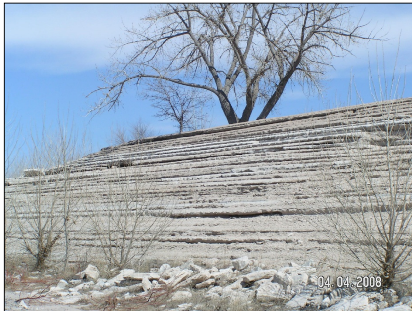
Figure 15. Bonny Reservoir Test Section after 57 years of exposure
