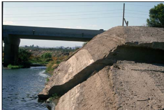
Figure 18. Displacement of Soil-Cement Bank Protection, north of Tucson, Arizona
