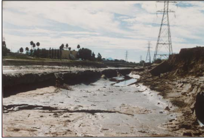
Figure 21. Overtopping of the Santa Cruz River Levee at Tucson
