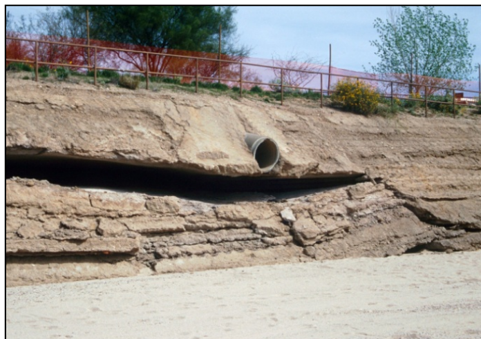
Figure 16. Soil-Cement Bank Protection on Rillito River, Tucson, Arizona
