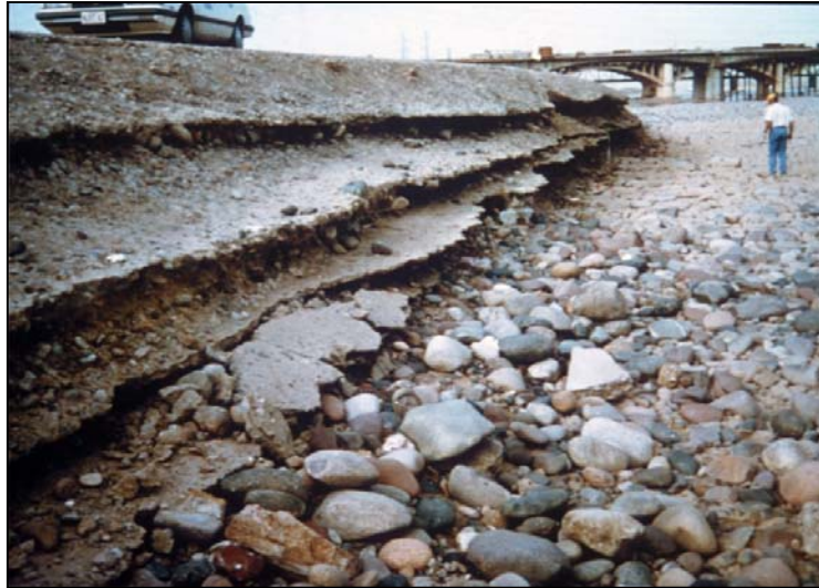
Figure 9. Scour of Cement Stabilized Alluvium along Salt River at Tempe, Arizona
