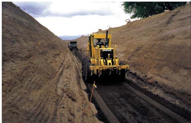
First lift of soil-cement being spread at elevation of maximum scour depth.
