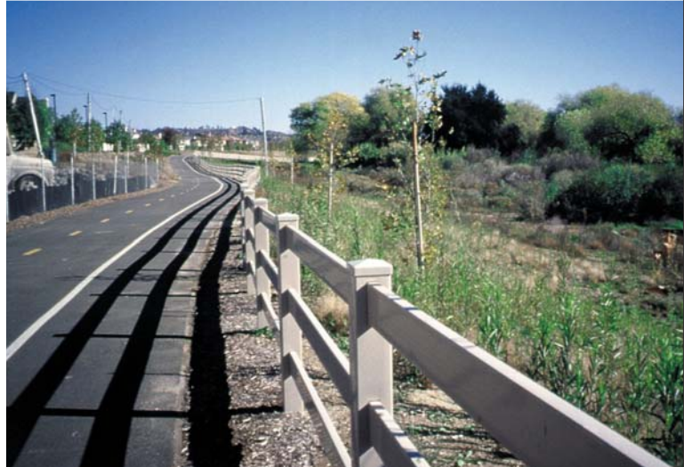
View of completed bank stabilization. Soil-cement is buried beneath recreational trail and landscaping.
